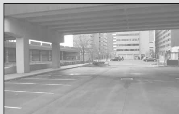
Underneath the MLK overpass. This section must be addressed in all design submissions. Photo by Danny Mayer.
